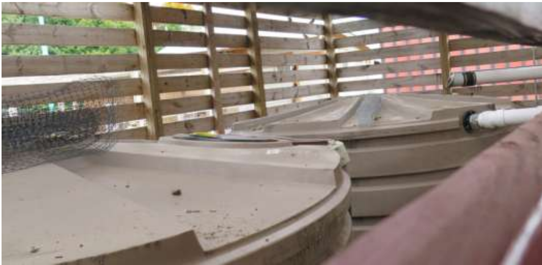
Water Collecting Cisterns
